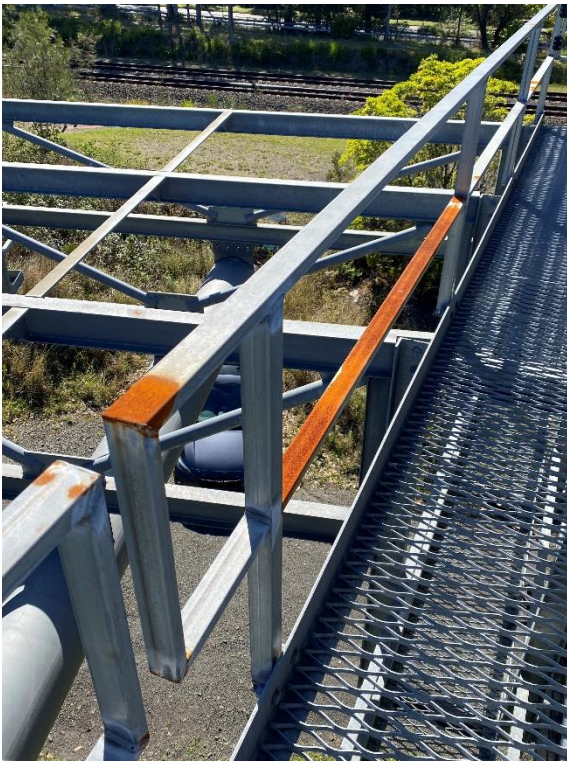
Photo 19 - Surface corrosion to handrailing (inbound side).
