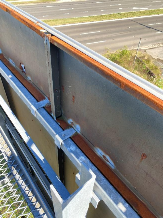
Photo 14 – Surface corrosion to signage pans.
