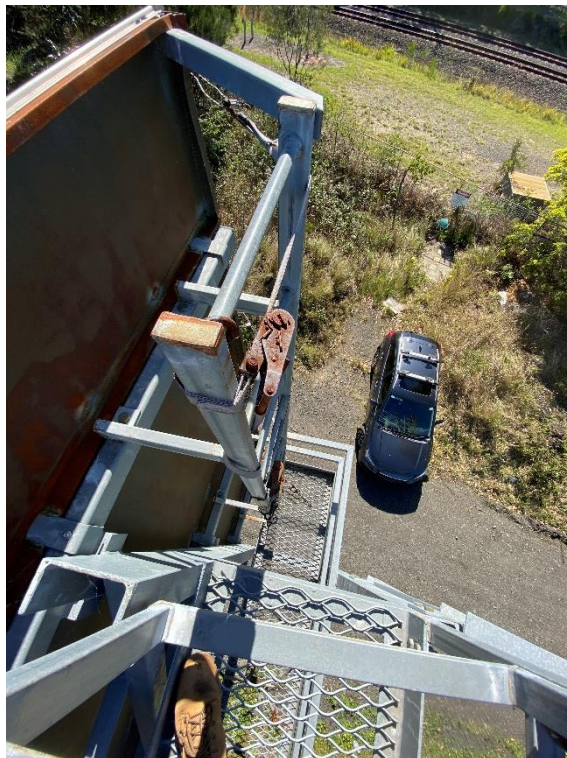
Photo 13 – Surface corrosion to gantry vertical ladder.
