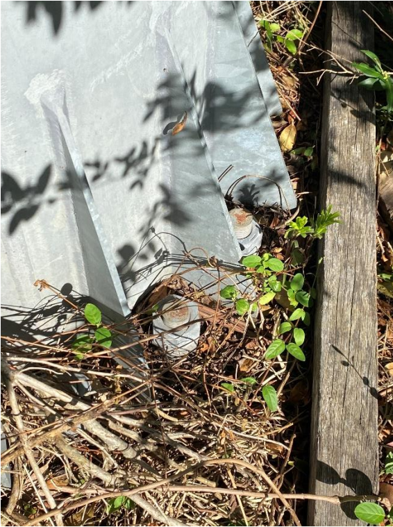
Photo 10 – Minor surface corrosion to hold down bolts.
