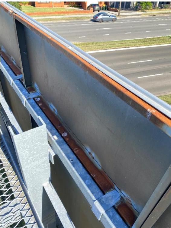
Photo 15 – Surface corrosion to signage pans.
