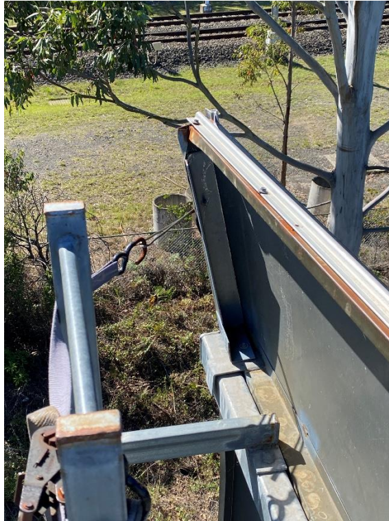
Photo 20 – Deformation to signage pan.
