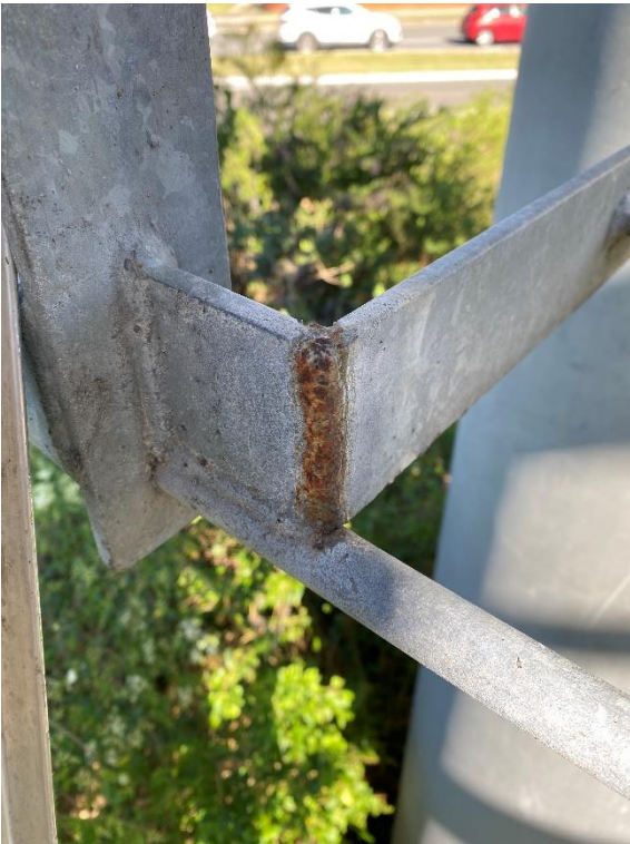
Photo 11 – Minor surface corrosion to vertical ladder support brackets.
