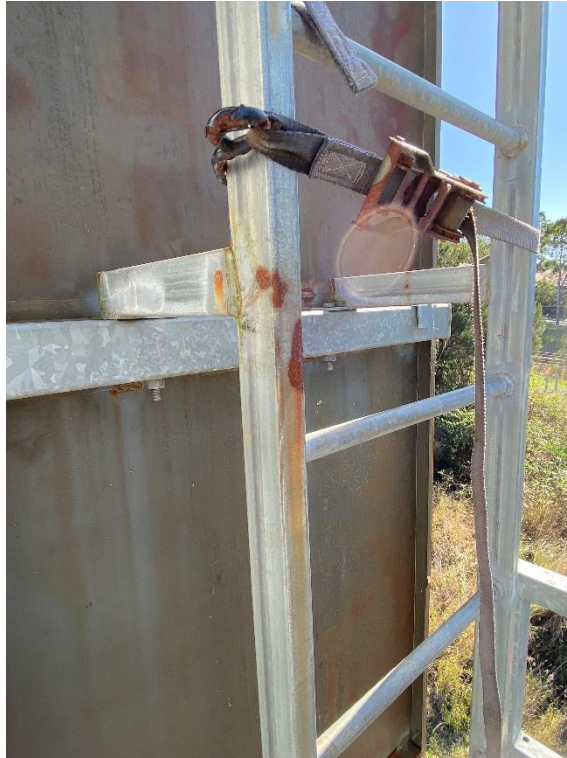
Photo 12 – Surface corrosion to gantry vertical ladder.
