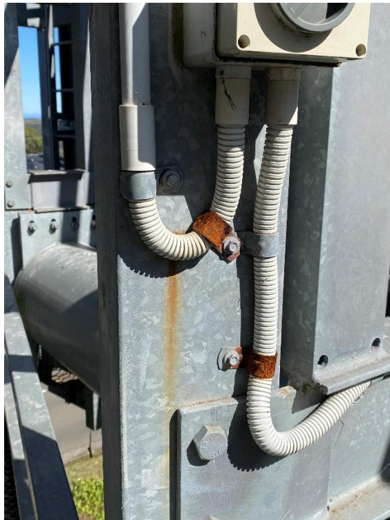
Photo 21 – Typical corroding conduit saddle brackets.
