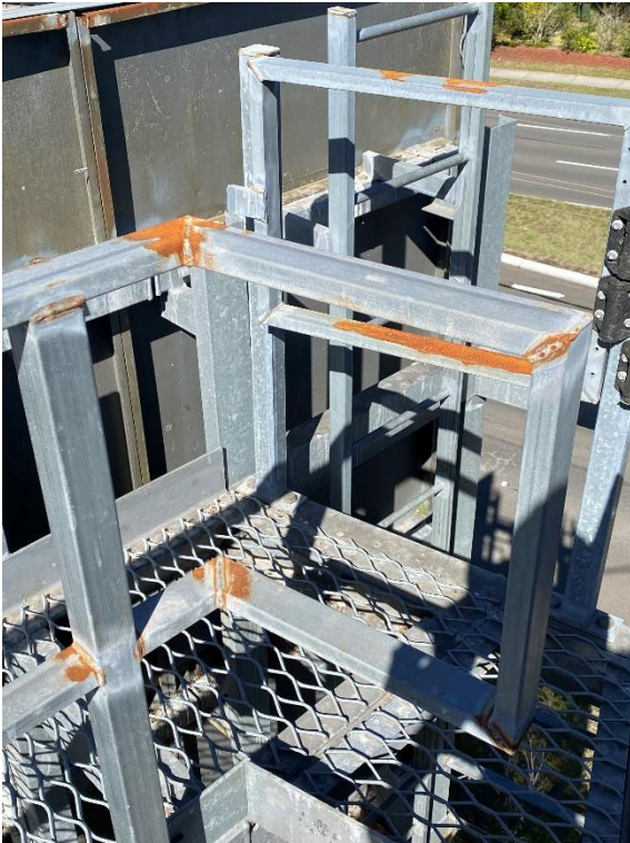
Photo 18 - Surface corrosion to handrailing (western end).
